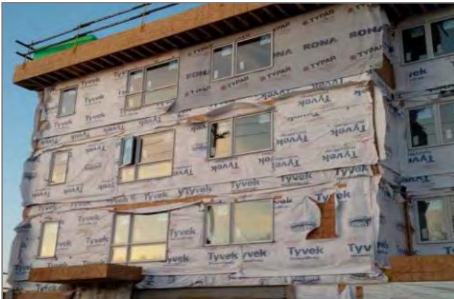
Figure 2.5 Poor House Wrap Installation
