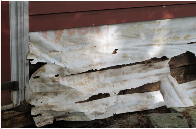
Figure 2.4 Photo of Building Paper after 30 years Behind Wood Siding.
