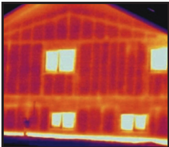
Thermal image of exterior framed wall showing heat escaping through the studs. Studs act as a thermal bridge through which heat can pass through the wall increasing heating and cooling loads.
