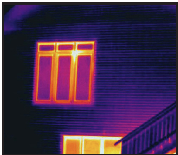
Thermal image of exterior LOGIX wall showing no heat escape through the wall. Continuous thick insulation with a solid concrete core wall prevents thermal bridging and heat escape through LOGIX walls.
