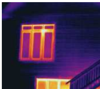
Thermal image of exterior LOGIX wall showing no heat escape through the wall. Continuous thick insulation with a solid concrete core wall prevents thermal bridging and heat escape through LOGIX walls.
